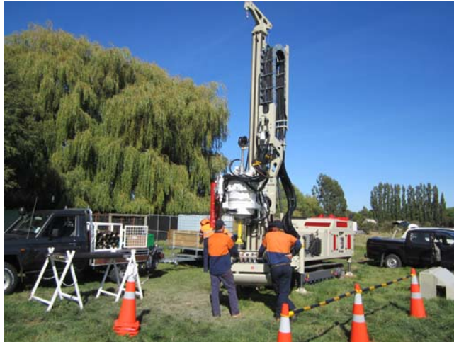
Drilltechniques' MC900P Comacchio drill rig, fitted with a Sonikor 50K drill head, working in New Zealand.
